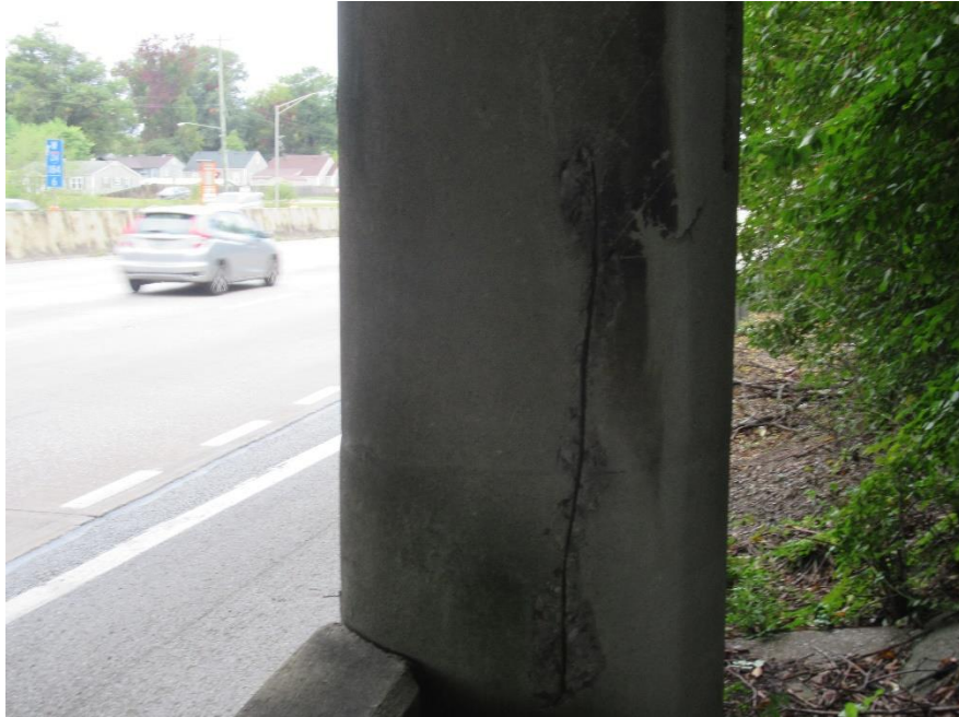
BENT #3 - COLUMN "A" - REBAR SPALL
