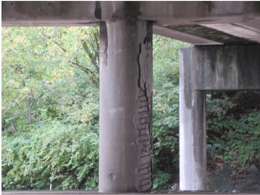
BENT #2 - COLUMN "B" - REBAR/SPALL/DELAMINATION
