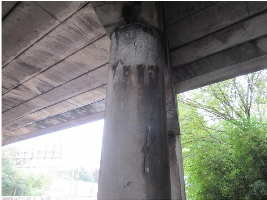
BENT #3 - COLUMN "B" - DELAM/SPALLS
