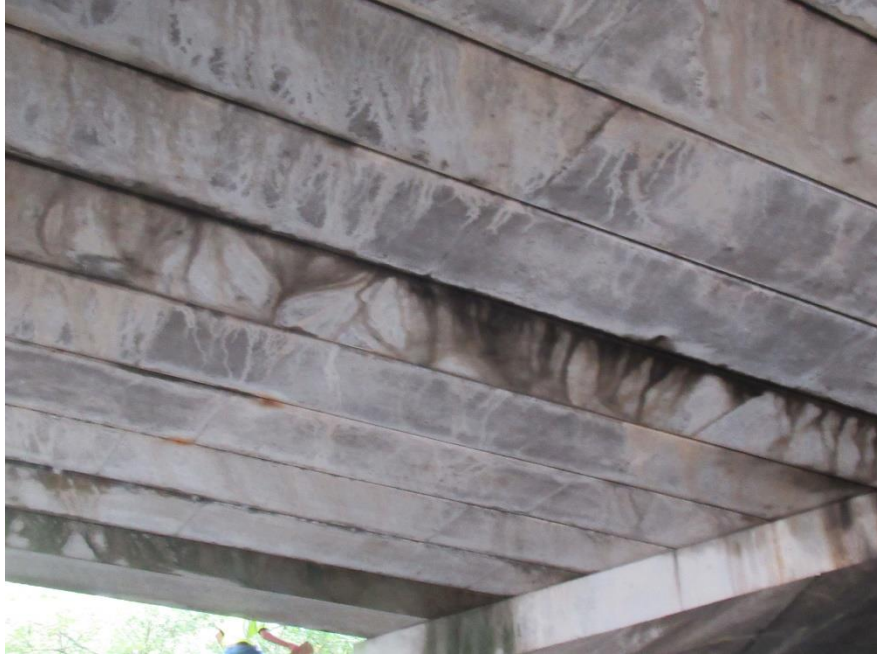
BOTTOM OF DECK - SPAN #3 - LEAKAGE
