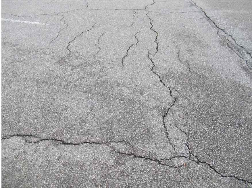
CRACKS IN WEARING SURFACE
