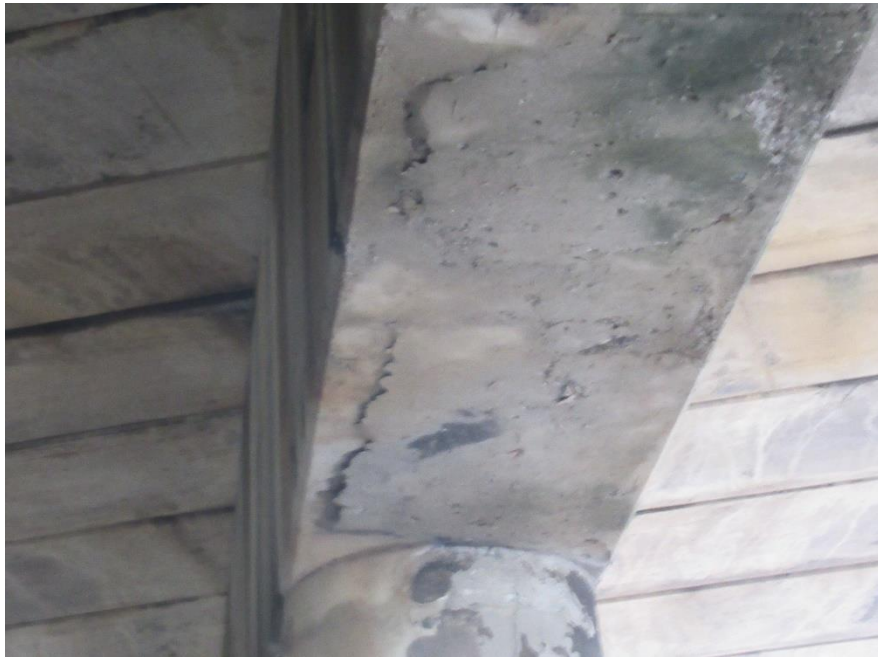
BOTTOM OF CAP - BENT #3 - BETWEEN COLUMNS - "B" AND "C" - DELAM
