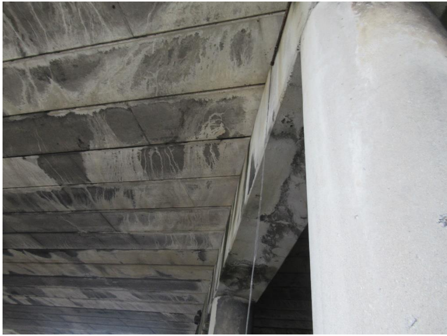
BENT #3 - COLUMN "E" - LOOSE ELECTRIC WIRING
