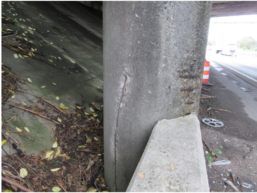
BENT #1 - COLUMN "F" - REBAR/SPALLS
