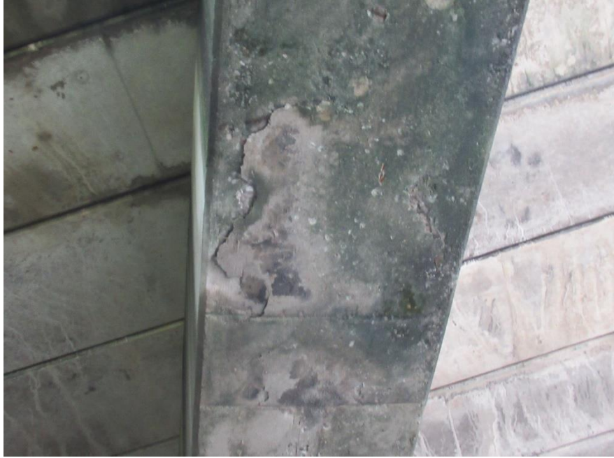
BOTTOM OF CAP - BENT #3 - BETWEEN COLUMNS "A" AND "B" - DELAM
