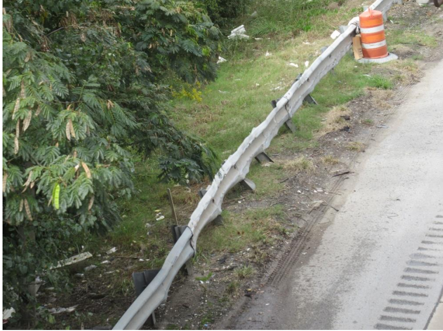
UNDERPASS EASTBOUND - #1 RIGHT - DAMAGED GUARDRAIL
