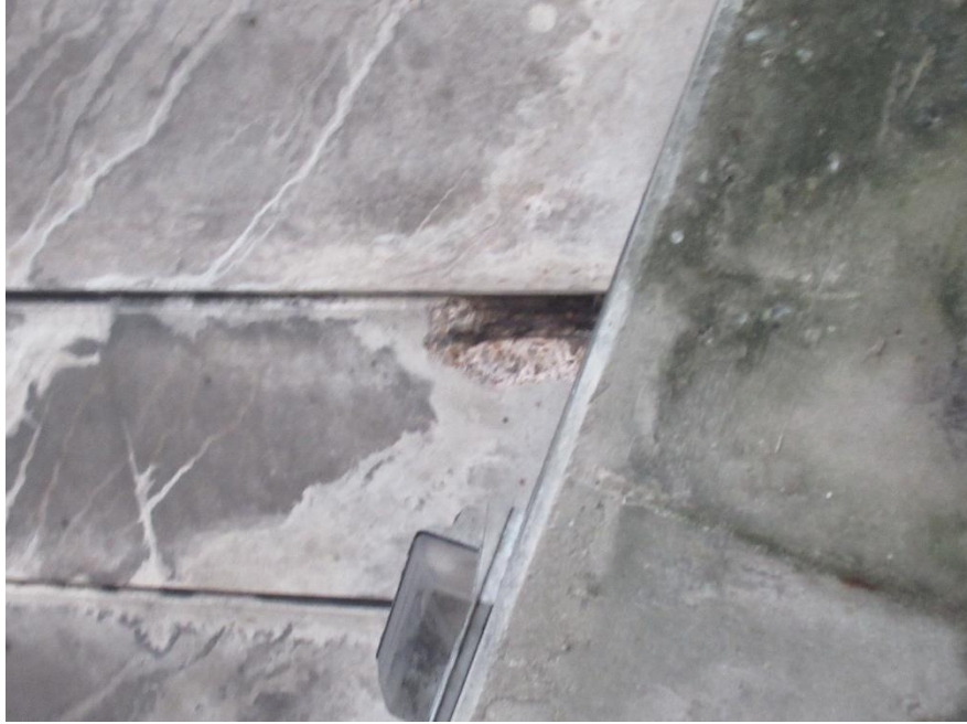
END OF BEAM "F" SPAN #2 - SPALL/REBAR
