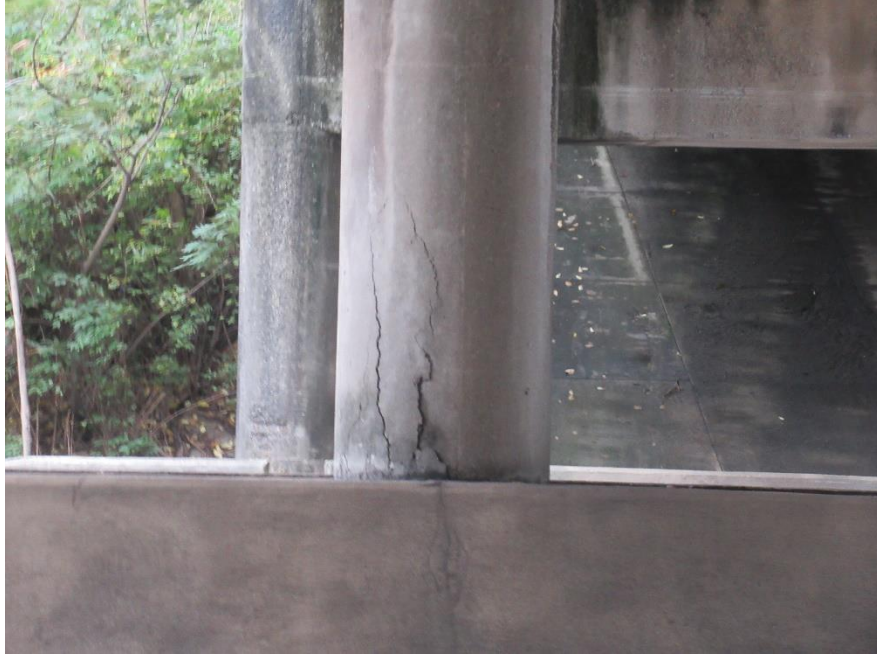
BENT #2 - COLUMN "E" - DELAMINATION
